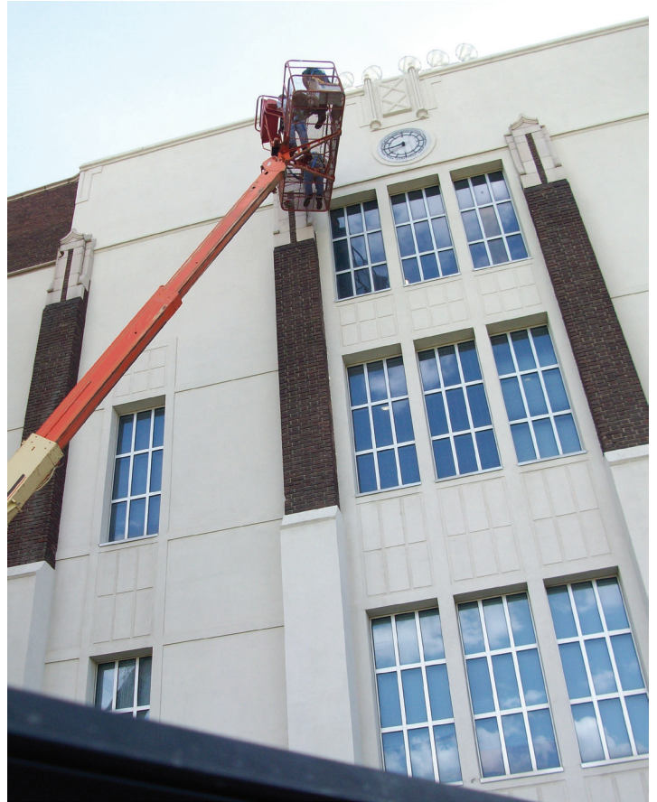
Sealing bat entry points in a school. Photo: Salt Lake City School District.
